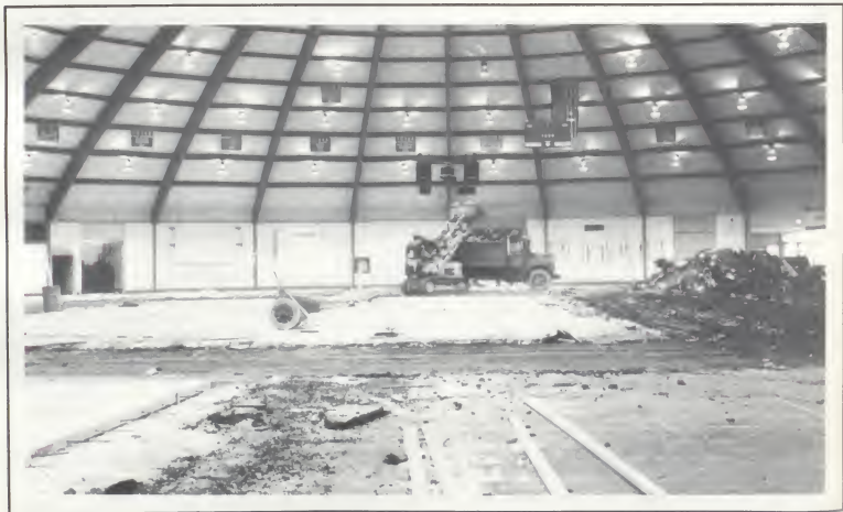
Long Gone. This vast emptiness will soon transform into a modern day facility to meet the needs of the community, thanks to the architectural expertise of Fanning Howey Associates, Inc., Michigan City. Congratulations to the Class of 1980.
